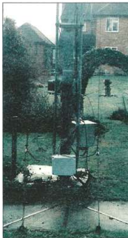
Termination of three wires of an 80m system, on a 18m versatower. The weatherproof box contains all components to switch, match and feed the array.
